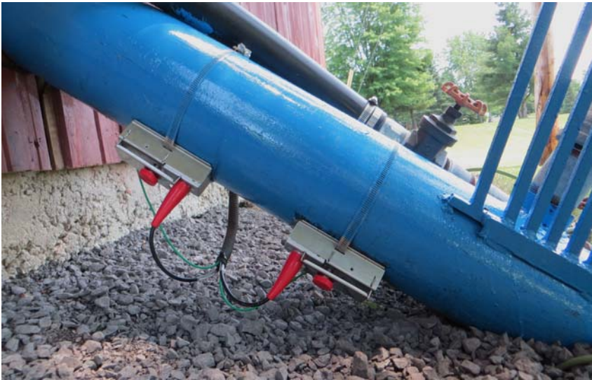
Clamp-on Ultrasonic Transducers Installed on 6" Steel Water Pipe
